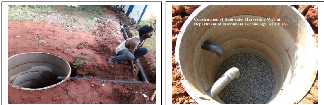
Figure 9 (a): RWH Well and Laying of Pipelines for Rainwater Harvesting at Department of Instrument Technology.
