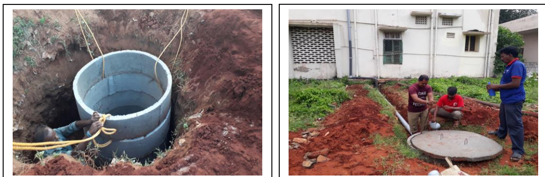
Figure 9 (b): Laying of Rings and Connecting the Wells with the Roof Top Rainwater Collection System.
