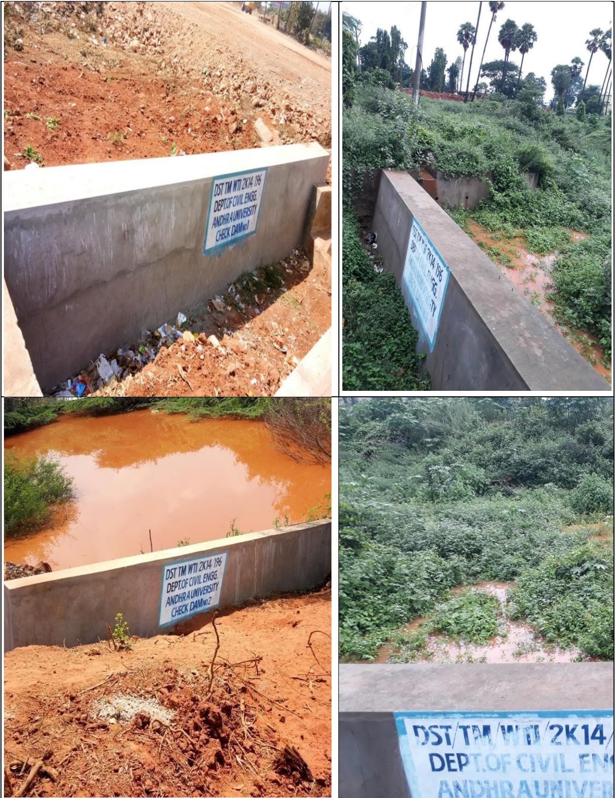
Figure 11: Check Dams Constructed in the Andhra University Campus as part of the RWH Program
